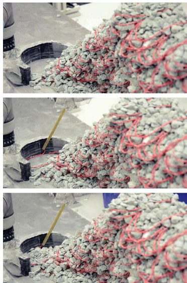
Fig. 12 Sequence of the fabrication process showing two six-axis industrial robotic arms equipped with customized end-effectors that cooperatively manipulate crushed gneiss and position textile strings according to a digitally generated weaving pattern. This is used for the robotic extrusion of textile strings that provide the lateral tensile support needed for preventing the buckling of the force chains and to stabilise the boundary fragility of the jammed structure (picture interval approx. 30 s.). Gramazio Kohler Research, ETH Zürich, 2014.
