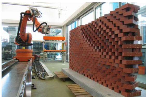
Fig. 4 Detail view of a dry-stacked automatically fabricated brick wall [19] together with a robotic setup equipped with a custom end-effector. Gramazio Kohler Research, ETH Zürich, 2006.
