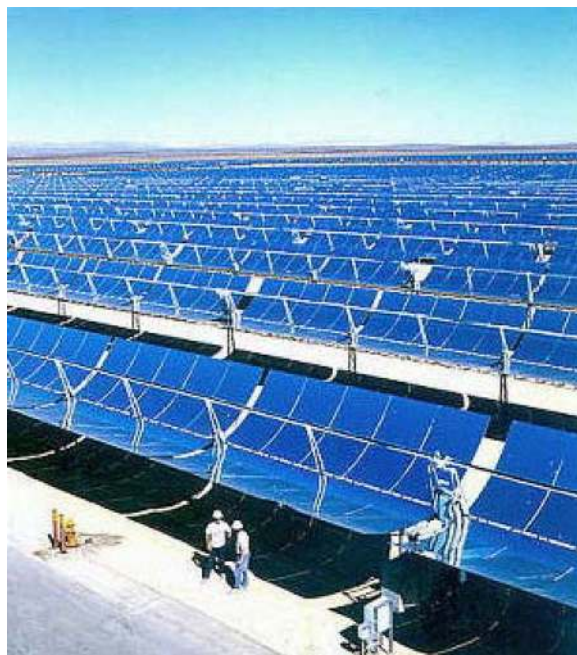
Fig. 3. The Solar Energy Generating Systems (SEGS) solar trough farm at Kramer Junction, California. The concept is that the reflective troughs focus sunlight on a pipe containing oil in a closed-cycle, which heats water to create steam to turbines. In total there are nine SEGS farms, with two at Dagett, five at Kramer Junction, and two at Harper Lake; all in California's Mojave Desert. The total area occupied is 2.4 sq km, generating 354 MW of power. These figures scale up to a footprint of 320 km by 320 km, if we were to supply 15 TW with this method. The nine plants have gradually been installed from 1984 to 1990, demonstrating over 20 years of performance without malfunction. Source: Power Corp.
