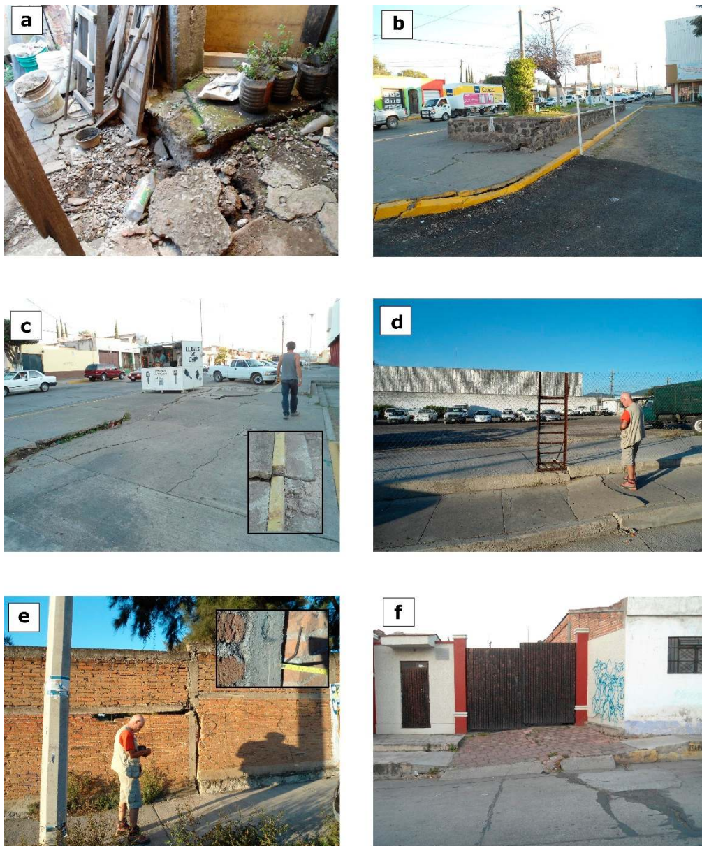
Figure 4. Photos showing evidences of ground fissures and faulting: (a) deformed and fractured pavement (site 1); (b) crossroads and sidewalk showing the pavement displaced and partially repaired (sites 3 and 4); (c) sidewalk affected by normal fault with a minor strike slip offset, as visible in the inset (site 5); (d) parking affected by fissures and normal faults (site 6); (e) sidewalk and wall affected by normal fault associated with a strike slip offset, as visible in the inset (site 10); and (f) street, sidewalk and gate affected by normal displacement (site 11). For the location, see Figure 3.
