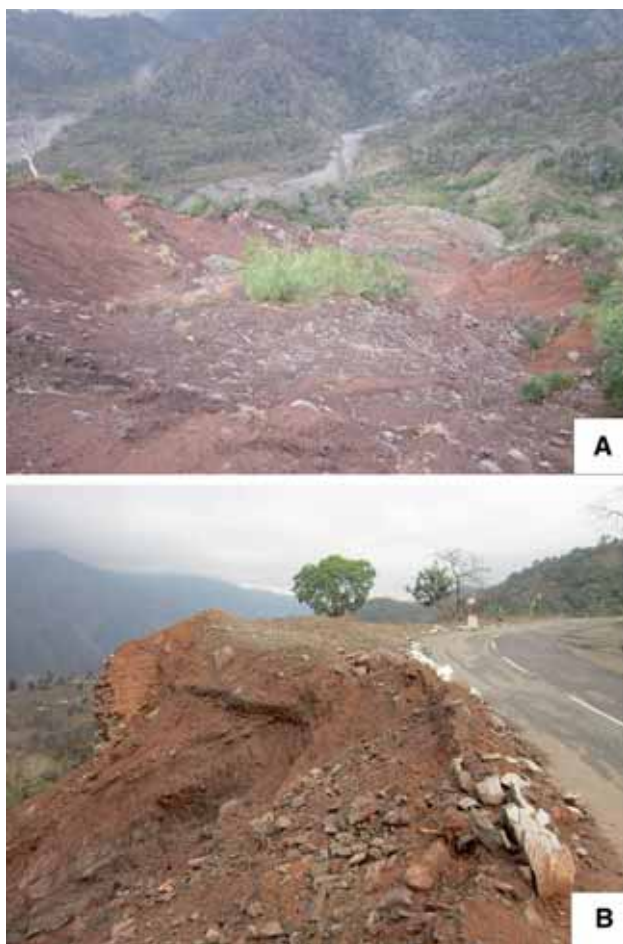
Figure 6. Field photographs of the Umri landslide in Haryana, India. The crown area is still unstable, causing serious damage to road.
