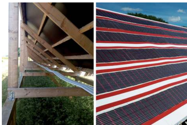
Fig. 1 Photograph of the wooden scaffold structure of the solar park installation (left) with six solar cell module stripes mounted on top of PVC plates (right).
