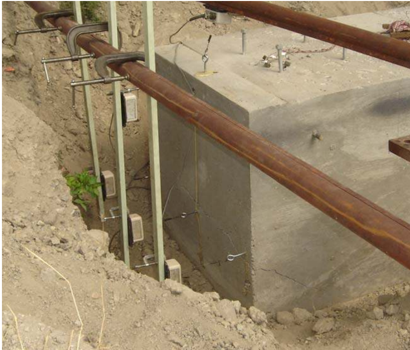
Figure 5-12 Initial cracking on the front face and size of Pile Cap 3.
