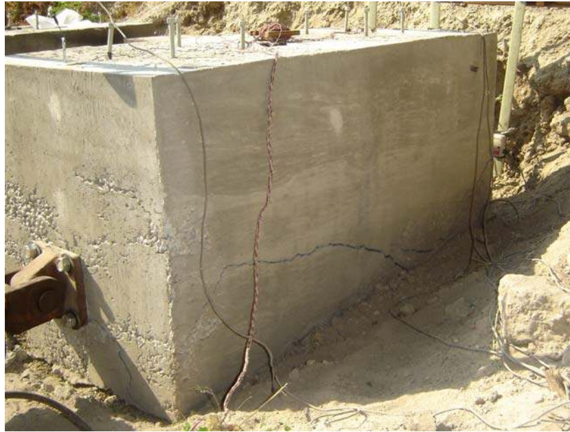
Figure 5-13 Cracking at a 90 kip load on the back and side of Test Cap 3.
