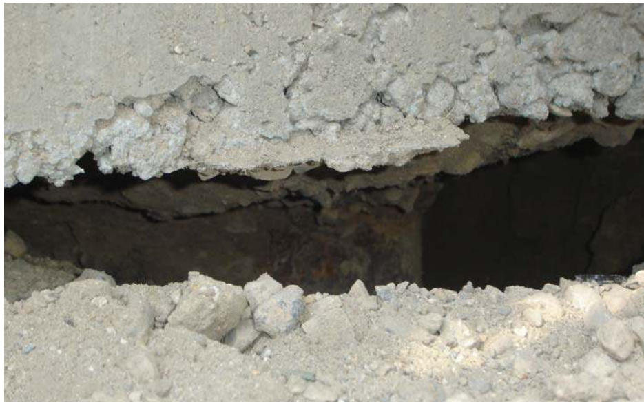
Figure 5-11 Test Cap 2 failure in pullout.
