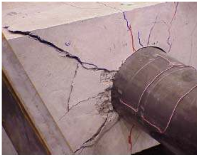
Figure 4-2 Failure of pile caps tested at Montana State University.
