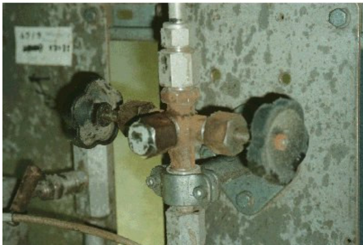
Figure 17 Corroded aluminium isolation plates and steel valves.
