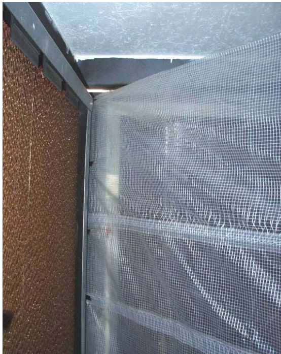
Figure 3-31 Plastic blocking device for cooltowers
