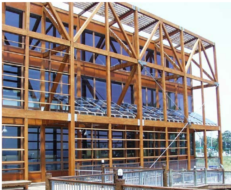
Figure 3-37 PV array and shading caused by CBF building structure
