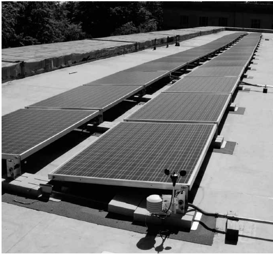
The 12-Kilowatt photovoltaic panels on the roof of the Hayden Library at M.I.T. look impressive but provide less than one percent of the library's daily electrical needs.
