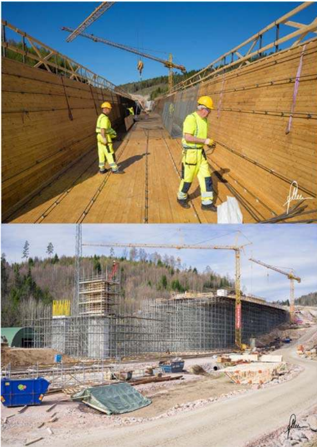
Fig. 2 Formwork and scaffoldings for Karlsnäs Bridge under construction (photographed by Patrik van Meer)
