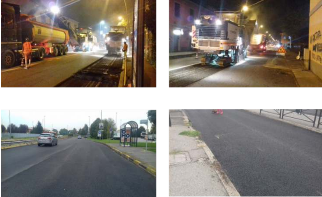
Figure 3: Works for the laying of new low-noise road surface in Viale Libertà (September 2018)
