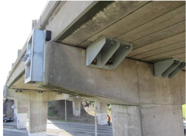
Figure 16: Pre-earthquake seismic improvements to bridges on Highways 73. (Photo credit: Craig Davis).
