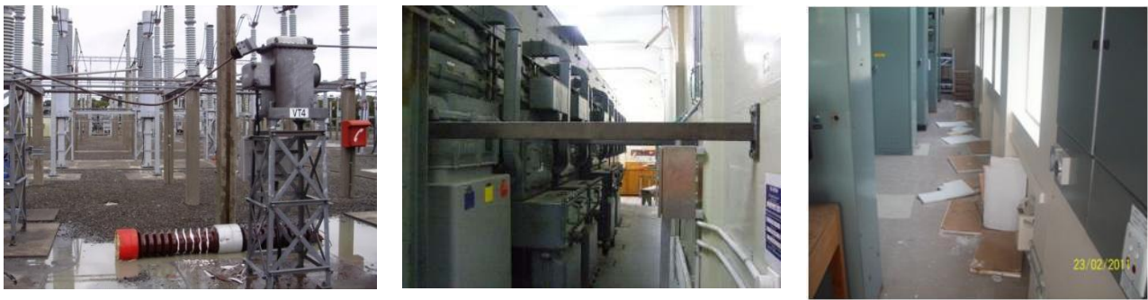
Figure 5: Bromley Substation: a) 220 kV failed current voltage transformer; b) Bromley bracing installed at the front and rear of the switchgear panels; c) dislodged ceiling tiles in the control and relay building, (Photo credit: Transpower).
