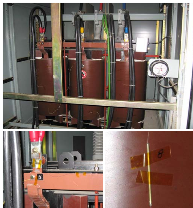
Figure 1. Application of FBG temperature sensors to high-voltage mold type transformers.
