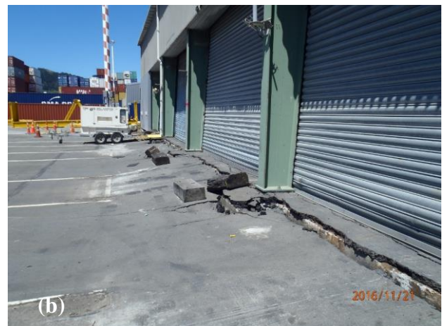
Figure 34: (a) Looking west across north wall of Building S37. Approximately 400mm of differential settlement between ground and deck of buried, pile-supported Pipitea Wharf that supports the western side of the shed. ( S41.278571^{\circ} E174.785632^{\circ} , 21NOV16); and (b) looking south along east wall of Building S37, which shows approximately 375 mm of differential settlement between fill and pile-supported east wall of the building. ( S41.279065^{\circ} E174.785787^{\circ} , 21NOV16).
