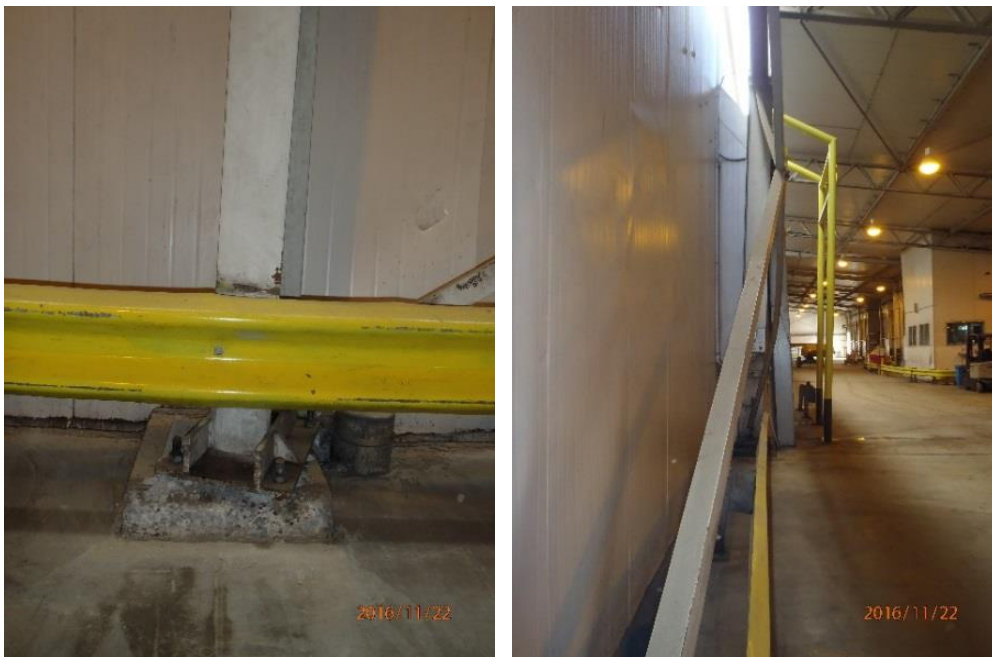
Figure 32: Internal east wall in northern part of the Shed, which shows column-pedestal connection failure due to rotation of the base of the column and buckling of concentric bracing. (Approx. at S41.280939° E174.784778°, 22NOV16).
