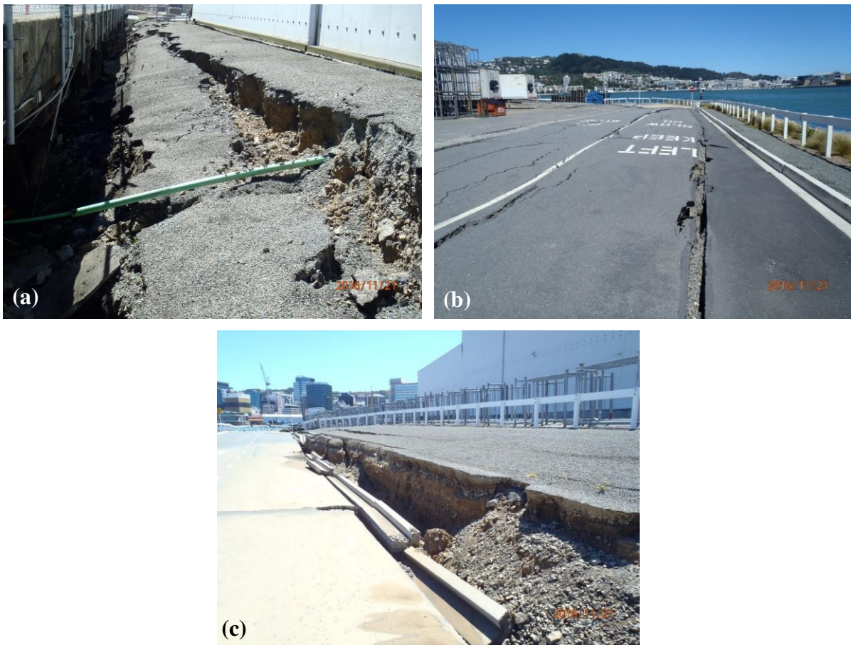
Figure 27: (a) Looking north along the west wall of the CS building. The ground settled approximately 530 mm relative to the pile-supported bulkhead of King's Wharf, which is shown at the left side of the photograph. (S41.280923° E174.784389°, 21NOV16); (b) Ground cracks in area west of the CS building and along the southwestern slopes of CentrePort (looking south). The CS building can be partially seen on the upper left corner of the photograph. (S41.281478° E174.784430°, 21NOV16); and (c) Approximately 1.1 m of vertical offset resulting from the southward lateral movement of the southern edge of CentrePort reclaimed land near its western side. Looking west near the southern wall of the CS building. (S41.281701° E174.785268°, 21NOV16).
