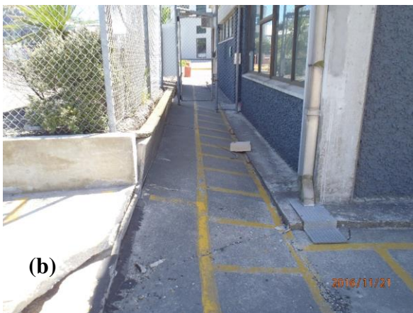
Figure 25: (a) Uniform settlement of CPH building which is founded on shallow foundations that apparently displaced downward the same amount as the surrounding fill. This photo is looking northeast at the southwest corner of the building. (S41.278395° E174.785639°, taken on 21NOV16). (b) Uniform settlement (230–260 mm) of the building relative to ground supported on the buried precast seawall that ran parallel to the bulkhead of partially demolished Pipitea Wharf. Looking north along western wall of CPH building. The perimeter walkway slopes down towards the building at 11 degrees over 1.35 meters. (S41.278395° E174.785639°, taken on 22NOV16).
