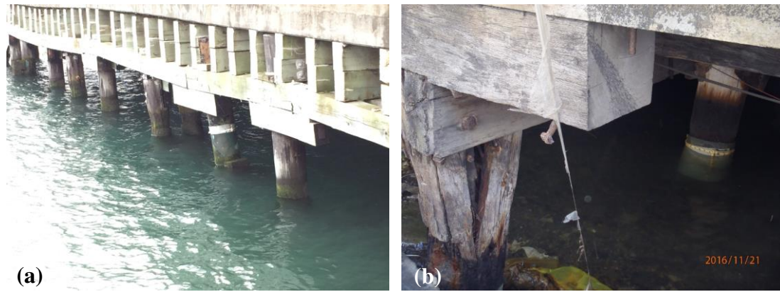
Figure 22: (a) Looking west along southern end of King's Wharf showing westward tilt of piles ( S41.281281^\circ W174.784097^\circ , taken on 17NOV16), and (b) looking under King's Wharf at an inland bulkhead pile; timber pile is split from lateral movement of the deck relative to the pile. ( S41.280900^\circ E174.784375^\circ , taken on 21NOV16).
