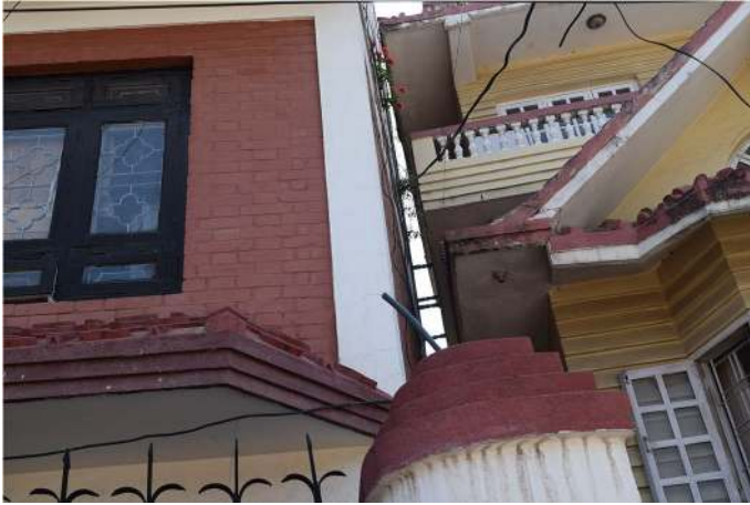
Fig. 12 Tilted building due to liquefaction at Imadol (Liq. ID 6 in Table 6) [Photo: RM Pokhrel]
