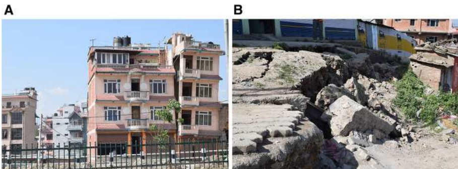
Fig. 5 a Partial collapse due to tilting and seismic pounding in the Kausaltar area (Location 7b in Fig. 2) after the Gorkha earthquake; b liquefaction and cracks in the ground near the Araniko Highway at Kausaltar, Bhaktapur, as a result of the Gorkha Earthquake 2015, (Location 7c on Fig. 2). Photograph taken on 2015-05-31 [RM Pokhrel]
