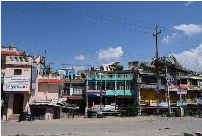
Fig. 15 Structural damage observed at Kalanki near Solti—no evidence of liquefaction (Liq. ID 10 in Table 6) [Photo: RM Pokhrel]
