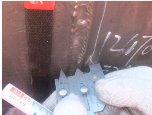
Figure 5. Profile of a mismatched weld joint.
