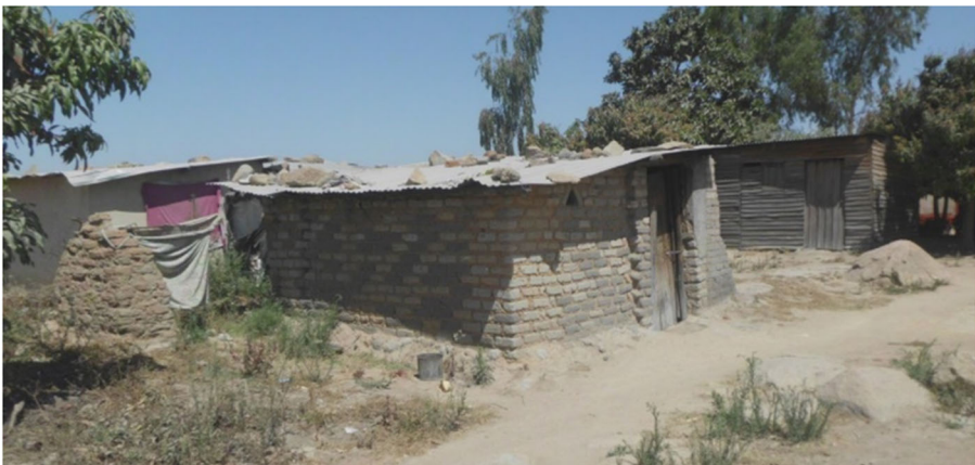
Fig. 4 Housing constructed with sub-standard farm bricks and the walls have been built using mud without cement. The roof is sagging in the middle showing a lack of trusses to support the iron sheets that are held in place by the bricks on top of the structure. In the background is a cabin made from wood that accommodates another family
