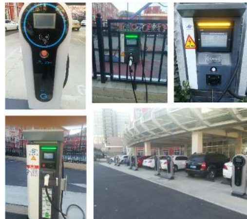
FIGURE 3. Charging station overview, including DC charging piles and AC charging piles.
