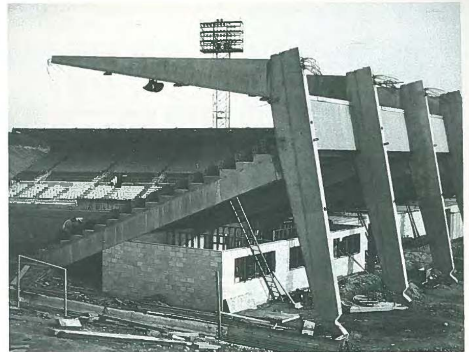
Fig. 68. Cheney Stadium in Tacoma, completed in 3½ months, did much to publicize the usefulness of prestressed concrete.
