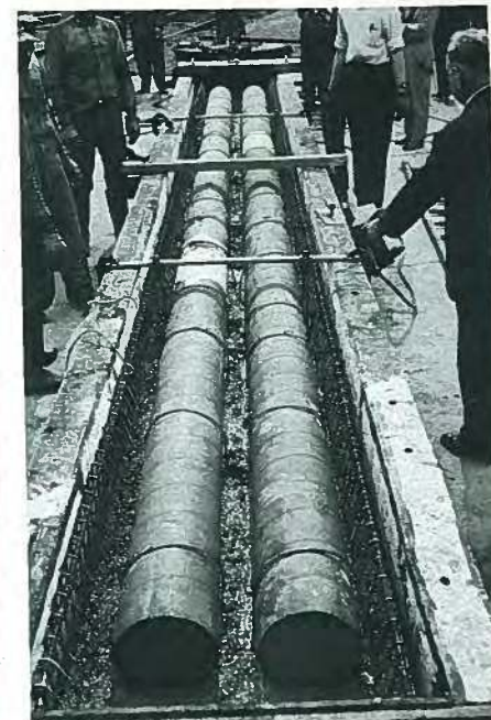
Fig. 20. Girder is about half cast, showing paper tubes used to form voids in the concrete.
