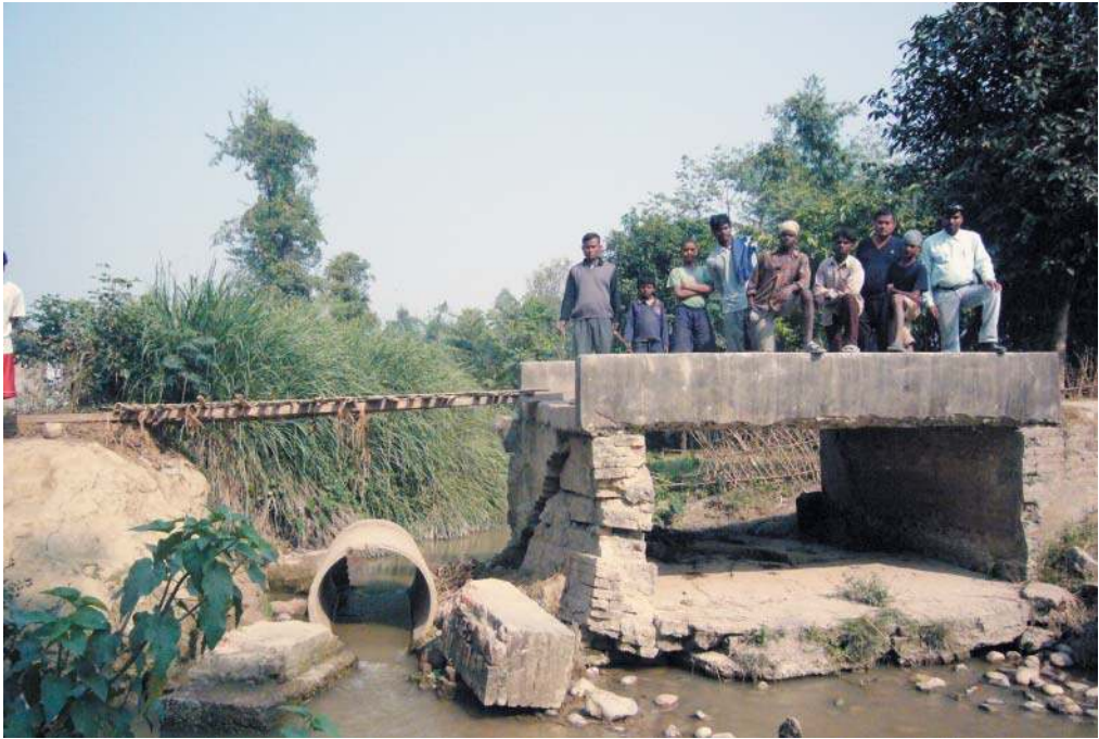
Local community standing on a bridge destroyed by flood, Singyali VDC, Mohottari District, Nepal
