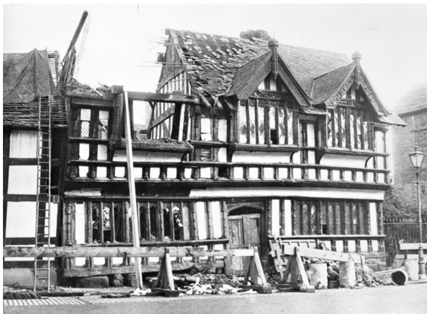
Figure 3: Bomb-damaged Ford's Hospital and adjoining listed building. David MacGrory, with permission.
