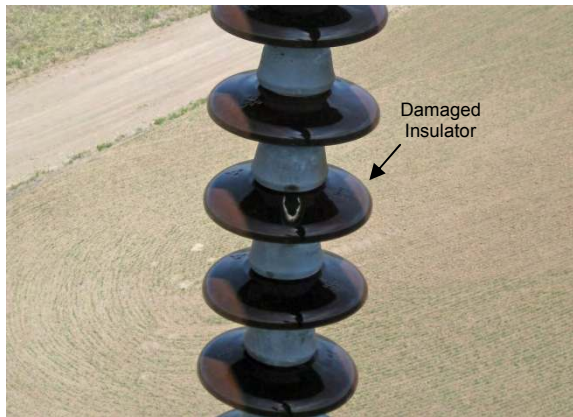
Fig. 26. Damaged insulator at 109.29 km from the Goshen terminal.
