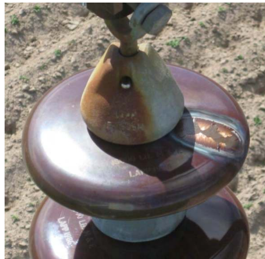
Fig. 34. Damaged insulator at 98.98 km from the Goshen terminal.
