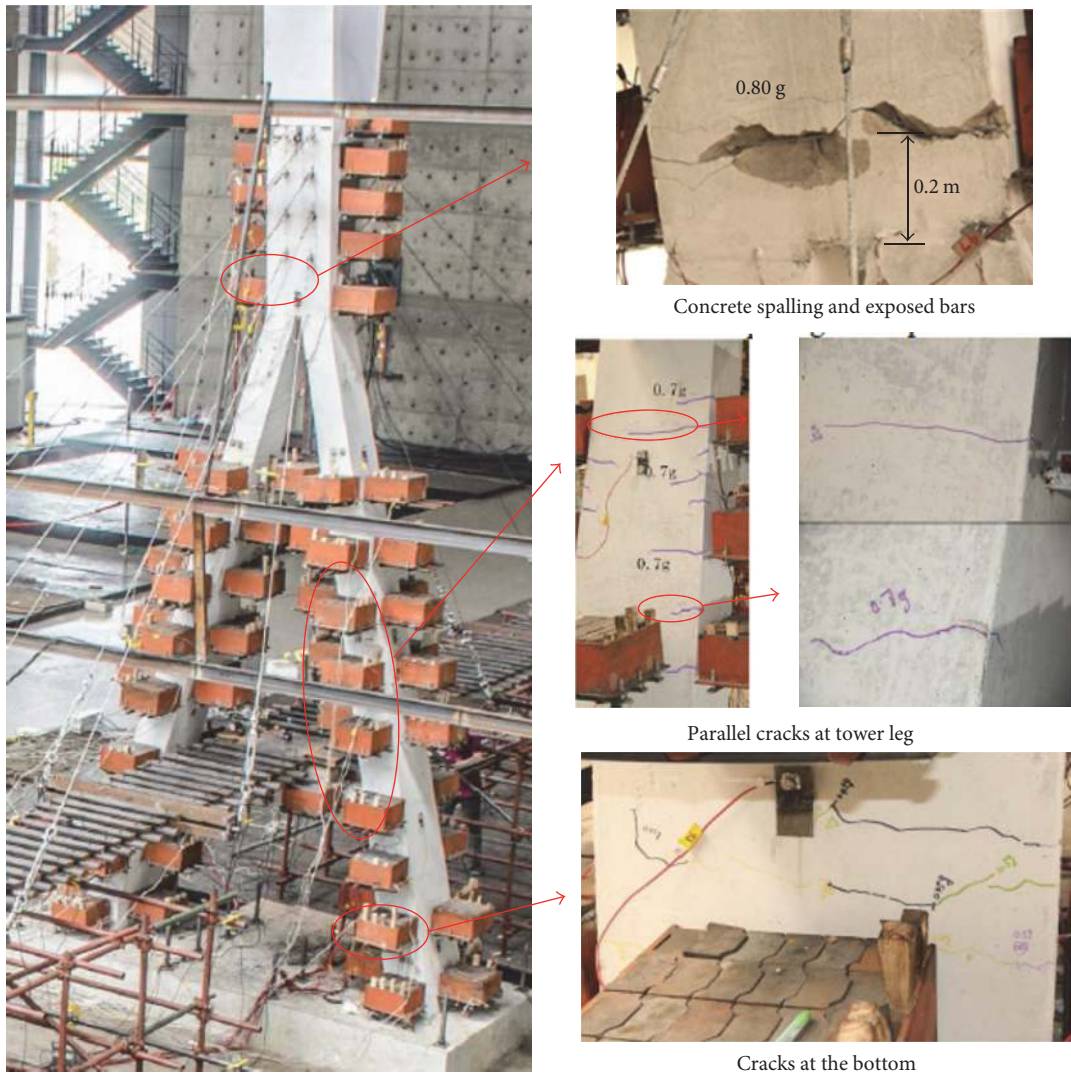
FIGURE 7: Observed seismic damage of the bridge model.
