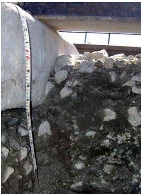
Figure 2-8: The ballast at the problematic mud pumping site is fouled with infusion of subgrade.
