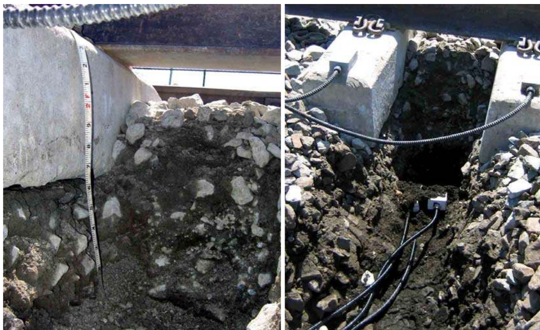
Figure 6-9: a) Fouled ballast between the concrete ties at the problematic area, b) Installation of sensors just below the fouled ballast.
