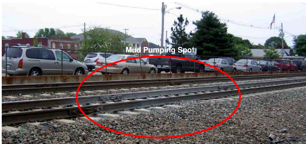
Figure 2-2: P2 - Mud Pumping Site at Mansfield. The mud pumping spot is visibly marked by white patches on the rails and concrete ties.
