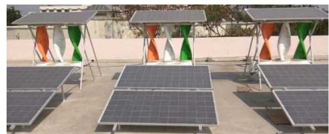
Figure 3. PV and Wind hybrid DERs installed in real-time
