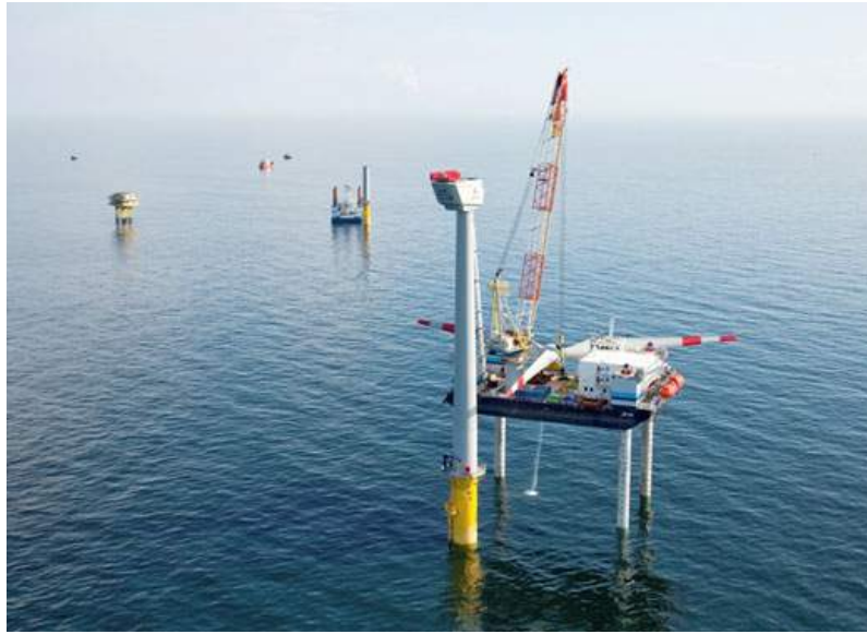
Figure 5.3: A jack up barge is used to replace or conduct maintenance on the rotor shaft or fan blades of a wind-turbine at sea.
