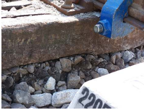
Figure 1.2: Severely worn ballast stones under an old sleeper. Compared with the new ballast stones nearby with sharp edges, the worn ballast stones have become rounded in shape and covered by dust. This problem is called the "foul" of the ballast, meaning that the ballast stones have been crushed, provide less drainage, move less, and have less elasticity, leading to a reduction in their friction dissipation.
