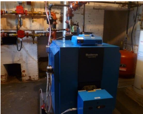
Figure 3.15: In the basement at Prescott House & Gardens Museum (Photo by the author, 6 October 2012).
