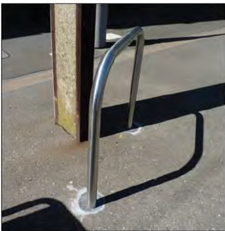
Figure 16.22: Rail placed too close to adjacent pole. (Source: author's own work.)
