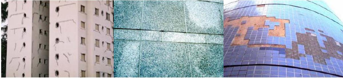
FIG 2: Different type of materials applied as façade coatings presenting anomalies.
