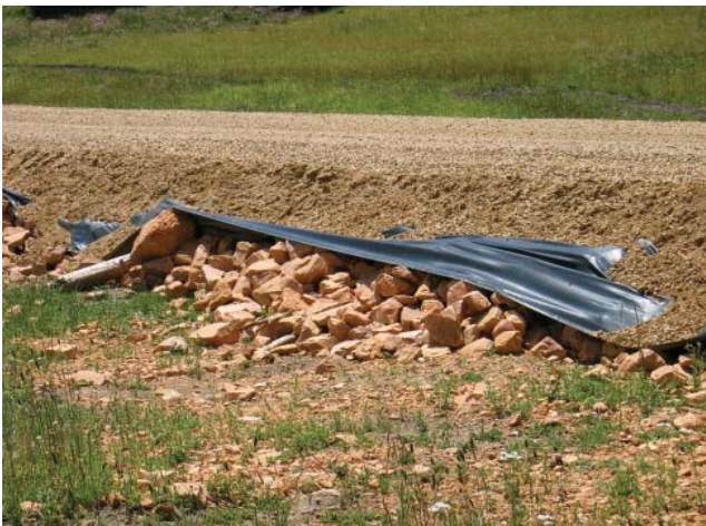
Geotextile is being used to strengthen this road through a wet area. Rock is laid on the wet surface, followed by geotextile and gravel on top.
