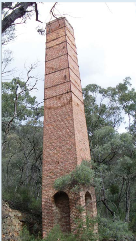
Chimney at the abandoned Tolwong copper mine, Ettrema wilderness, Morton National Park, Australia
