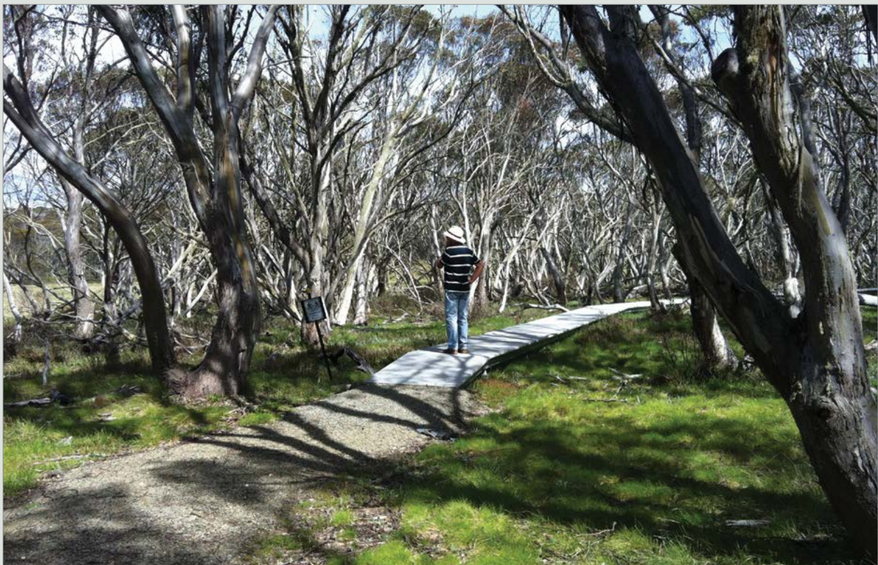
Elevated walkway built to protect a high-value Aboriginal place in the Alpine National Park, Victoria, Australia
