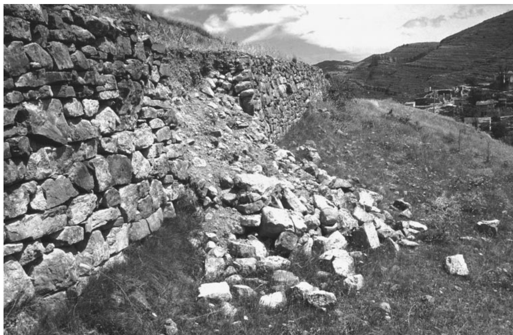
FIGURE 5 Collapse of a terrace wall at the foot of a hill near a village resulting from hydrological pressure higher up (Soto en Cameros, Leza Valley). Fields in this gently sloping area were only abandoned within the last 10 years. (Photo by L. Ortigosa)
