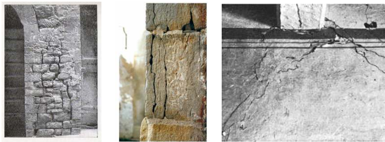
Figure 3. Crushing due to compression.
