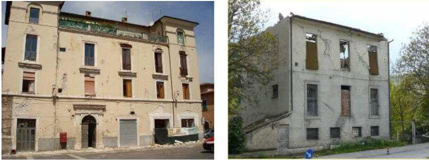
Figure 5. In plane failure due to compression and shear.
