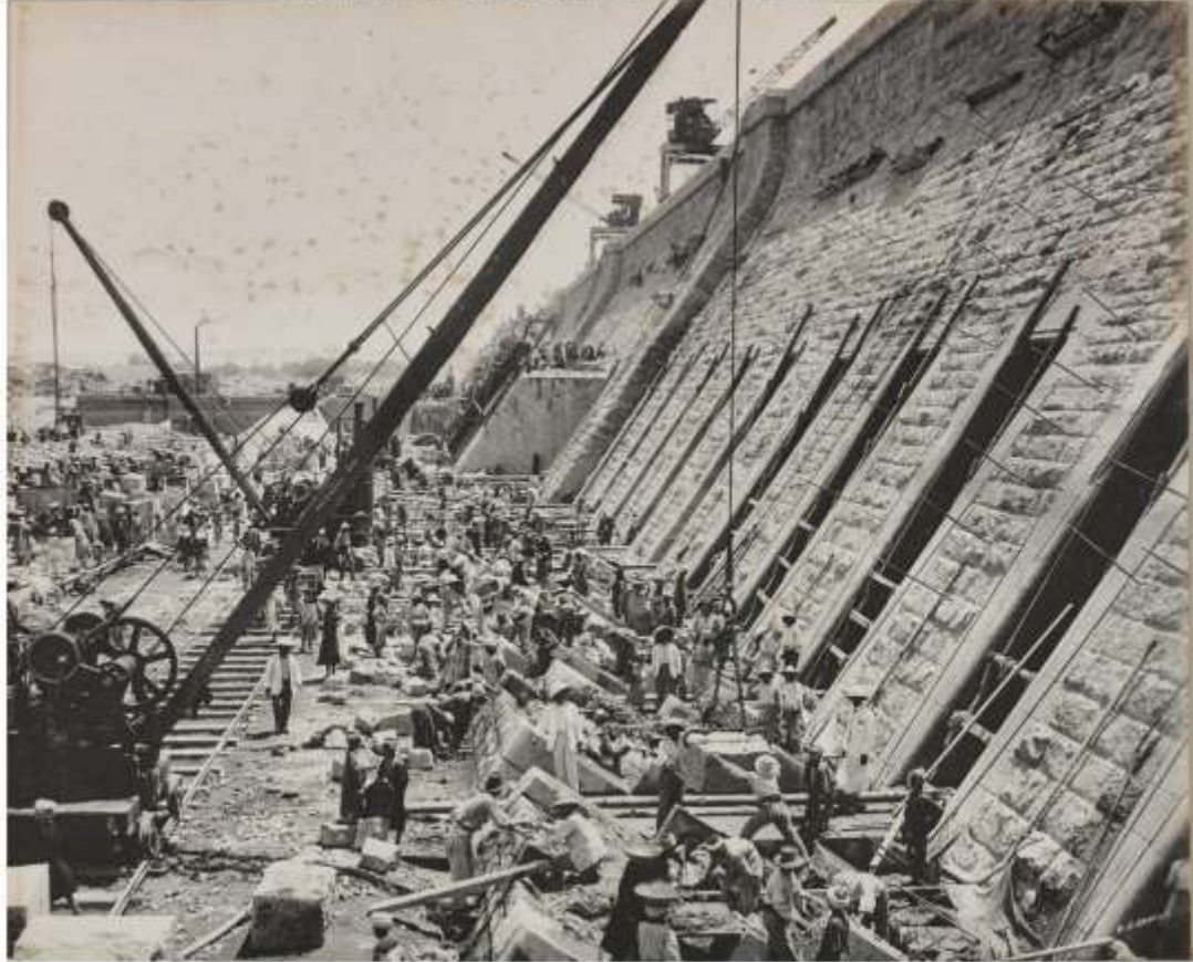
Figure 3 Top: "Aswan Dam: Excavation in progress at Bab-el-Kibir." HIL 455/8. Bottom: "Extending sluices in thickened portion of the dam." HIL 454/14.
