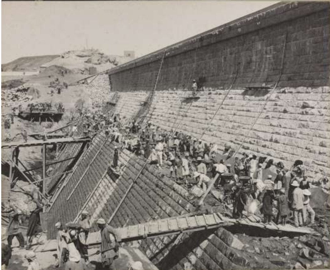
Figure 4 Top: "Aswan Dam: Commencing masonry in deepest part of foundations at Bab-el-Kibir." HIL 455/9. Bottom: "Thickening at solid dam." HIL 454/9.
