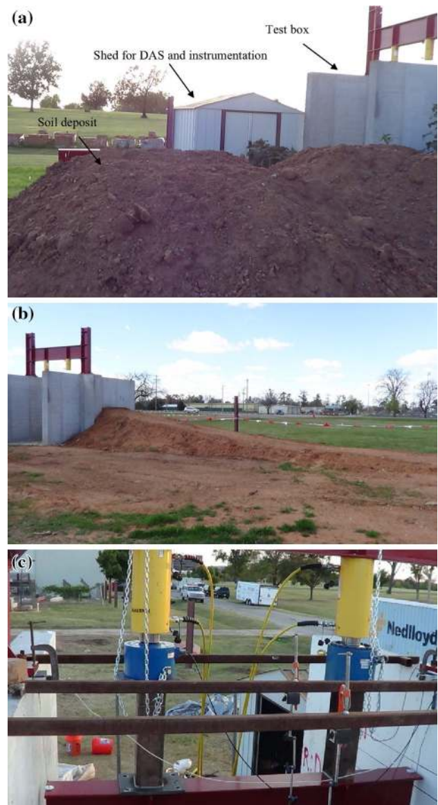
Fig. 1 a Large-scale outdoor test facility for reinforced soil walls and embankments at OU; b ramp for transporting soil to the test box using a front loader; c loading assembly
