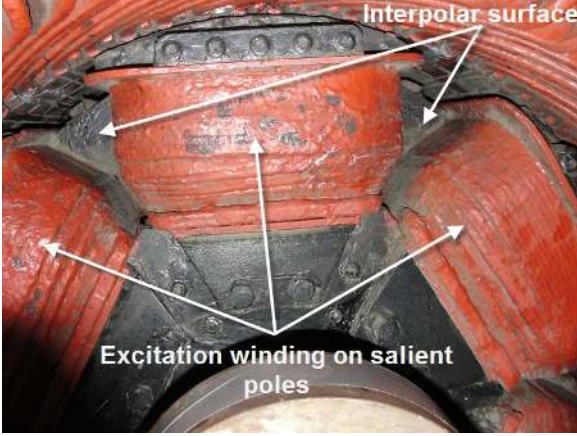
Fig.4 – View on the rotor of the observed generator
