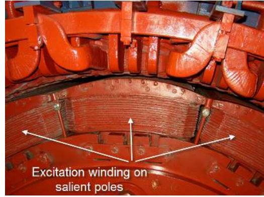
Fig. 8 - View on the rotor of the generator in Hydro Power Plant HE "Vinodol" ( o = 40 )
