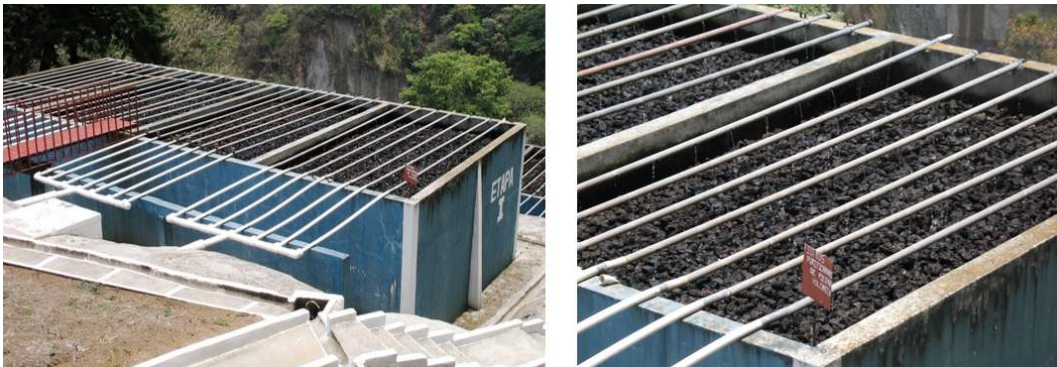
Figure 5. A volcanic rock trickling filter with a fixed hydraulic distribution system. This system has been in operation for 35 years with an average daily flow rate of 500 m 3 /day. Filter located at the University of San Carlos, Guatemala City, Guatemala (photo by Stewart Oakley)
