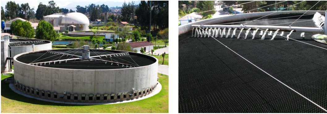
Figure 4. a) A plastic media trickling filter with a rotary hydraulic distribution arm designed for a flowrate of 40,000 m 3 /day (Cuzco, Peru). Note the ventilation ports around the base in the top photo. (b) close up of distribution system (photos by Stewart Oakley)
