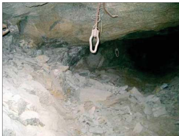
Figure 10—Pillar 14 and the fractured rock in the ASG after the burst
