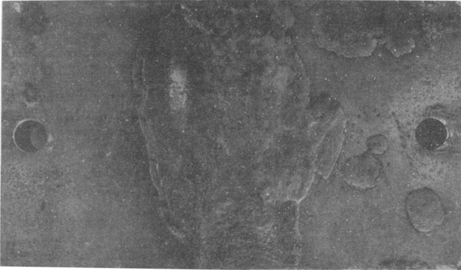
Figure 2. Corrosion products on the weld zone after one month of exposure at Tuticorin seawater.
