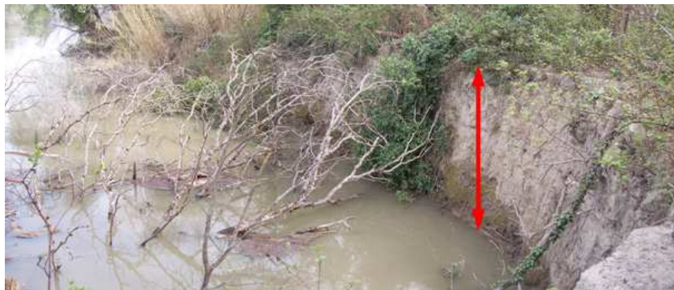
Fig. 8. Bank erosion. The red arrow represents the 3.5 m elevation gap seen on Fig. 7 (source Cemagref)
