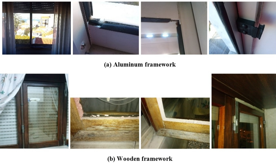
Fig. 8. Illustrative example of window frames near the end of their service life (a) aluminum framework, (b) wooden framework
