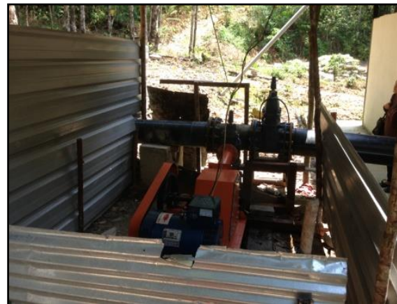
Figure 2(b). Power House.
