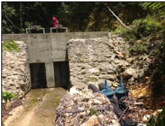
Figure 2(a). Installed Micro-Hydro System.
