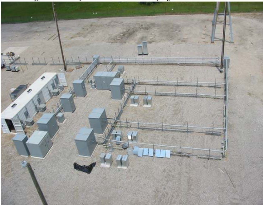
Figure 6. Layout of the CERTS Microgrid Test at the Dolan Technology Centre
