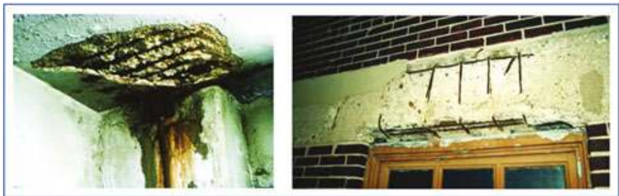
Figure 2. Deterioration of normal concrete [7].
