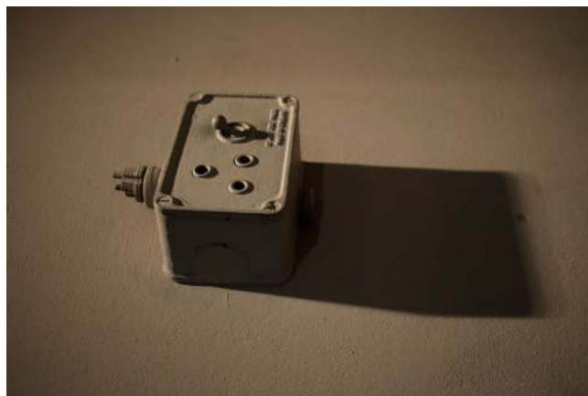
FIGURE 3 'When you have the one configuration it is a piece of home electronics, you just adjust it slightly and it becomes this other thing'. Light switch, Churchill War Rooms (Alexis-Martin 2018).
