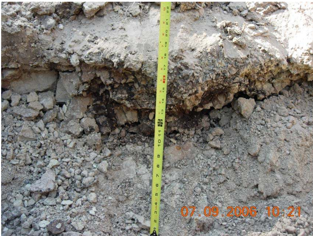
Figure A1 . Organic-Rich Zone in Subgrade Soil.
