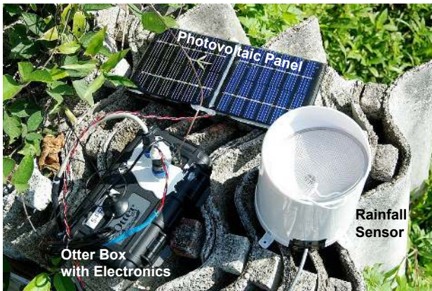
Figure 6: Rainfall Sensor Node Consisting of Electronics, Sensor, and Photovoltaic Board
