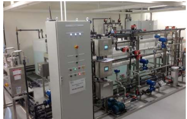
Figure 1: Secure Water Treatment (SWaT) testbed
