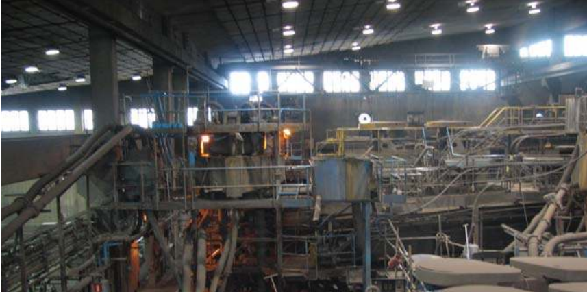
Figure 1.2: Wireless control of froth flotation process at Boliden within the SOCRADES EU project ( http://www.socrades.eu/ ).
